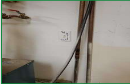
1.1 Shut off for boiler
