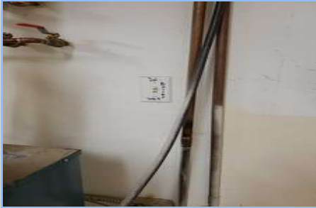
1.1 Shut off for boiler
