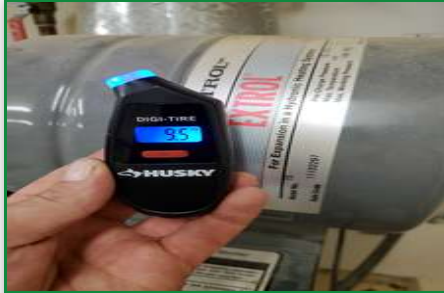
1.2 Pre system run PSI on expansion tank
