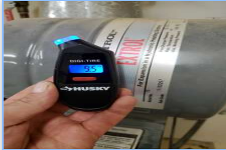
1.2 Pre system run PSI on expansion tank
