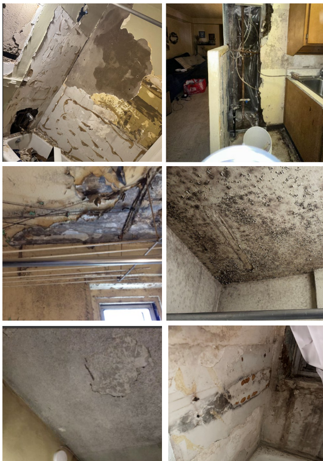
Examples of severe conditions in NYCHA apartments reported to the OCC in 2025.
