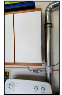
Renovate or Replace Vent System
