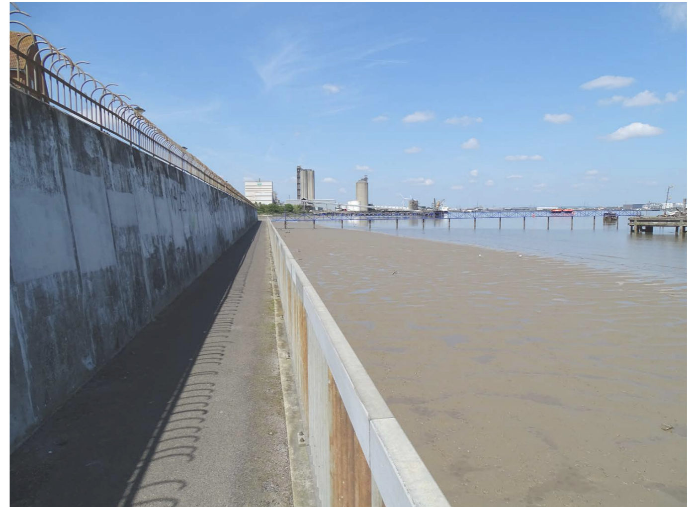
Thames Path next to Chandlers Drive, Erith. - Another section of path which lacks a physical connection with the existing housing making it feel unsafe.
