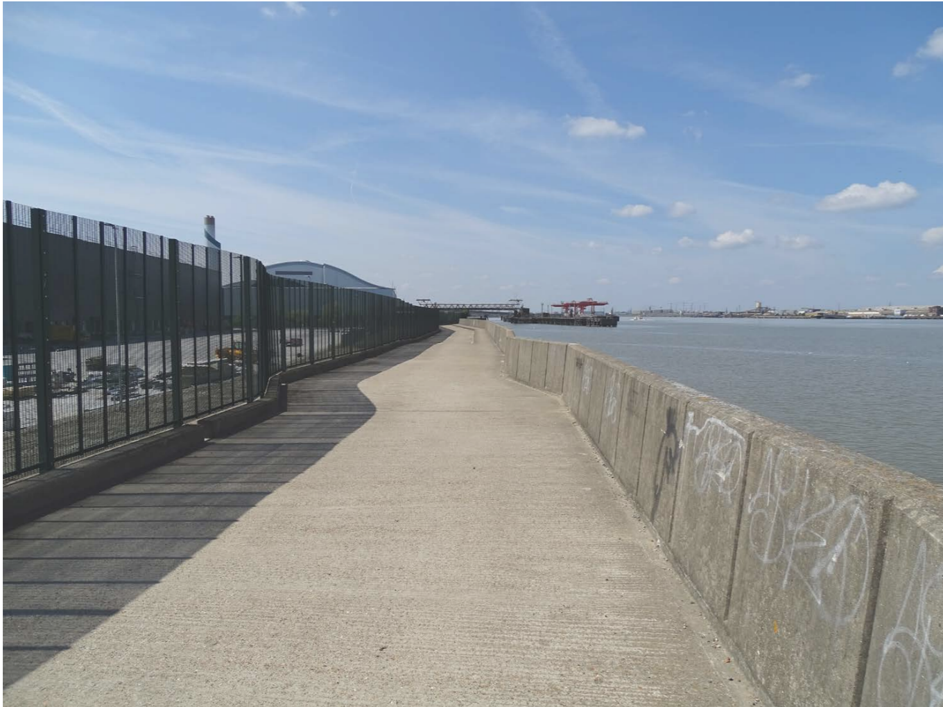
The path becomes wider and new metal fencing has been erected - Belvedere Industrial Estate.
