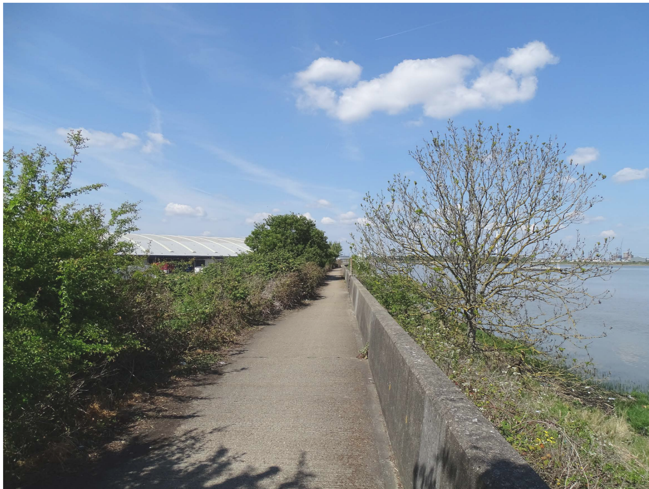
Path next to Lidl regional distribution hub, where nature is trying to regain control of the bank - Belvedere Industrial Estate.
