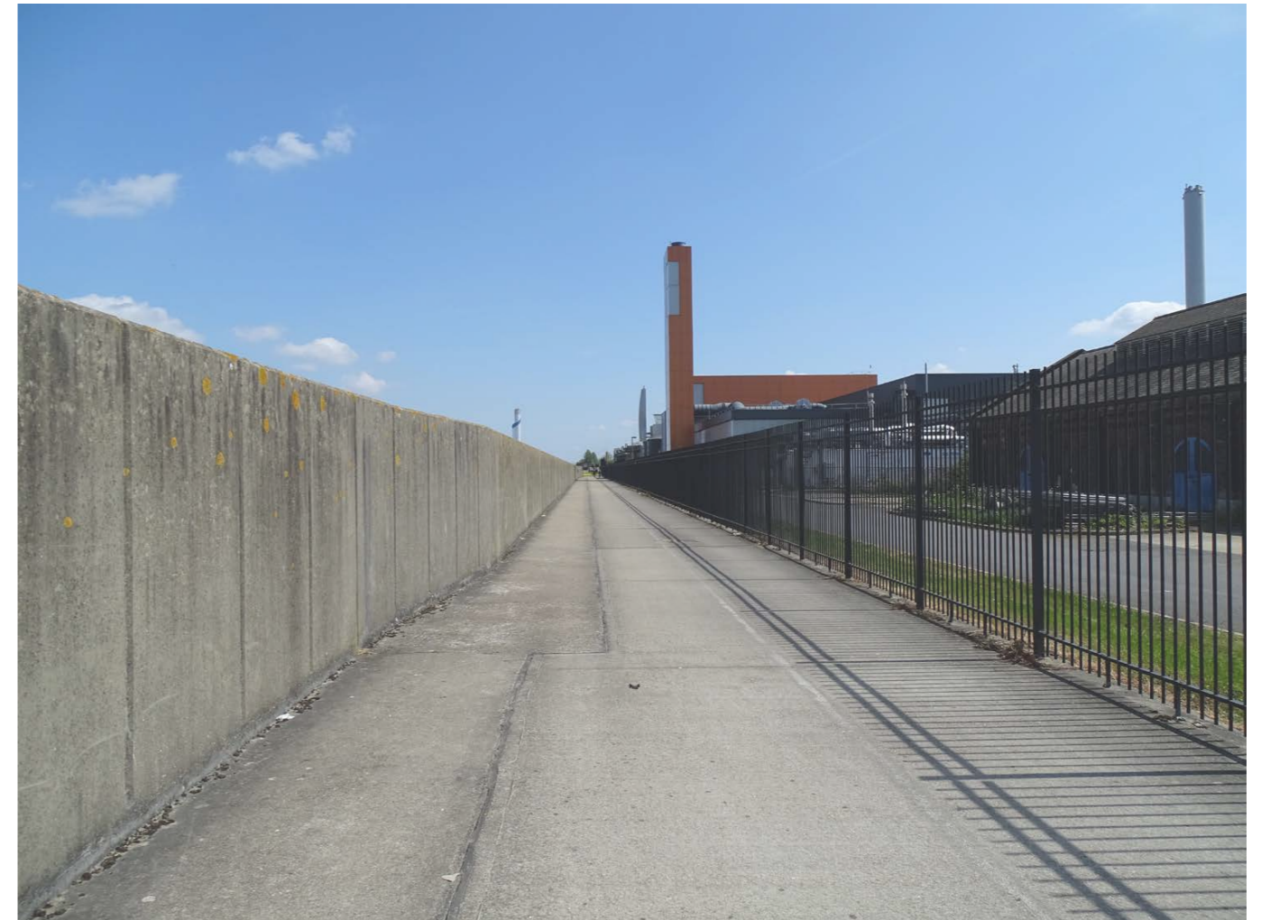
Concrete flood barrier wall - A blank canvas for artists to improve the view for cyclists and walkers.
