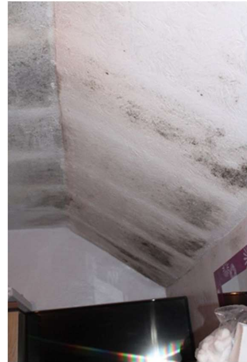
Lack of ventilation assessment
