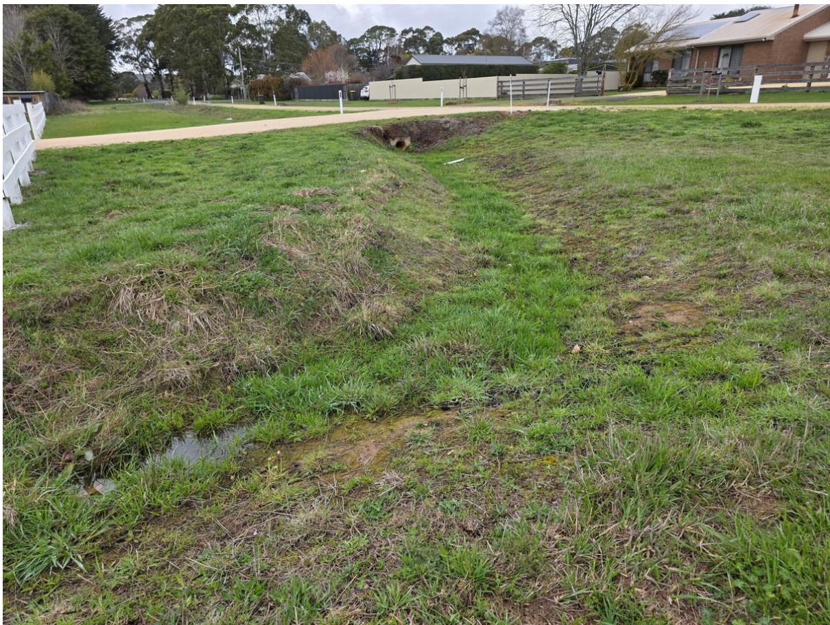
Plate 1 Drain in the south-east corner of the reserve that discharges into the drainage-line wetland
