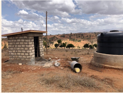
New pump house for the well. It will also be a power distribution point.
