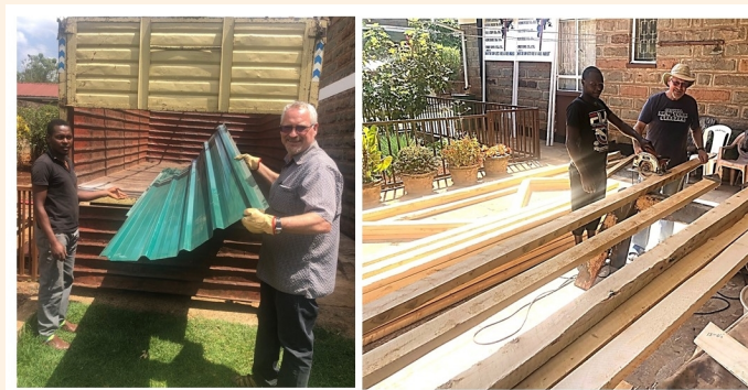
105 iron sheets have been purchased and all the trusses have been made for the Lokusero-B church!
