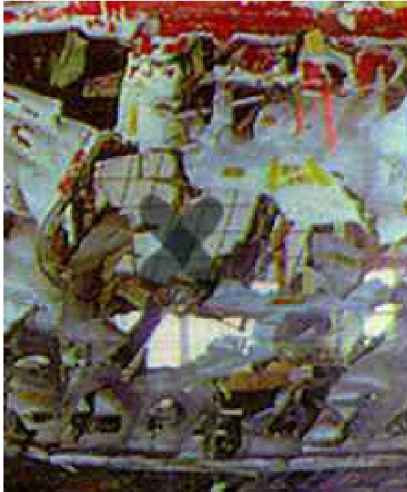
“X” marks the spot of the outward peeled rupture of the aft midspan latch of the forward cargo door of TWA 800. Note hinge and red paint smears on fuselage skin above shattered door.
