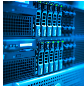
Servers and Routers
