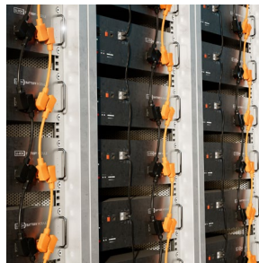
Energy Storage System
