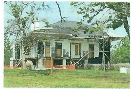
Beauvoir (April 2006), 7 months after Hurricane Katrina (before roof was repaired, without porches rebuilt).
