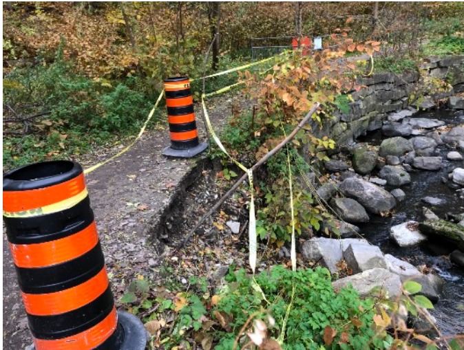
Retaining wall (previously just under rightmost yellow ribbon) undercut by Aug-Sept storms. Wall to north (built just before 1900) soon to go.
