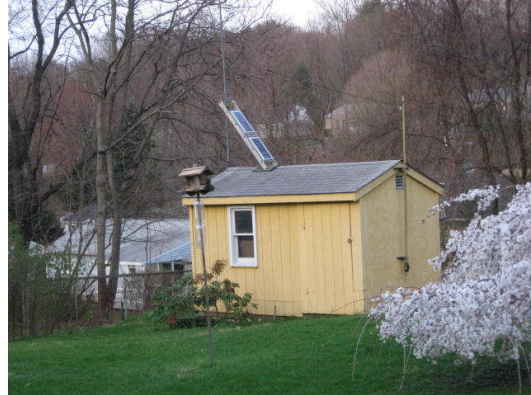
Solar array mounted on shed
