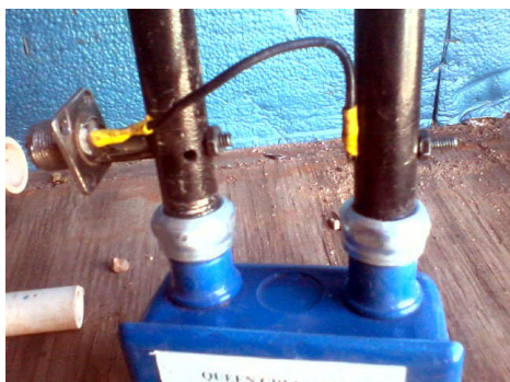
KB7KWK's modification of his original feed line attachment that is shown in the Superstition ARC newsletter (available at www.vailrd.net/qcejp.pdf ).
