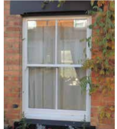
Sliding sashes in original timber tend to be replaced with plastic these days, but here Richard has made them in traditional styles, now using Accoya instead of tropical hardwoods, and modern essential machinery
