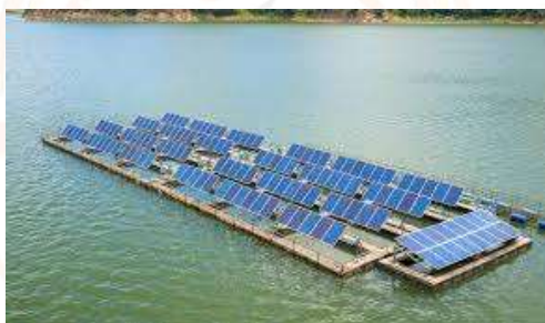
Floating Solar Solution
