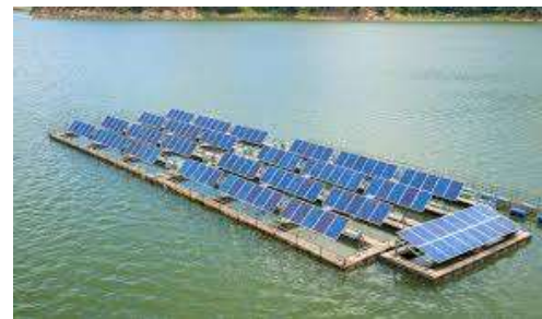
Floating Solar Solution
