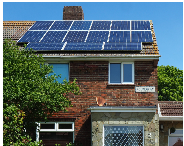
PV panels integrated into the roof of a dwelling within Coldean.
