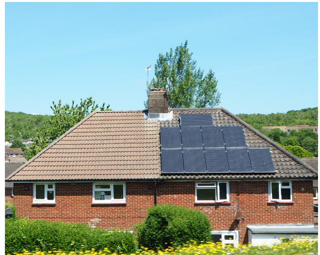
Solar panel retrofit within Coldean.
