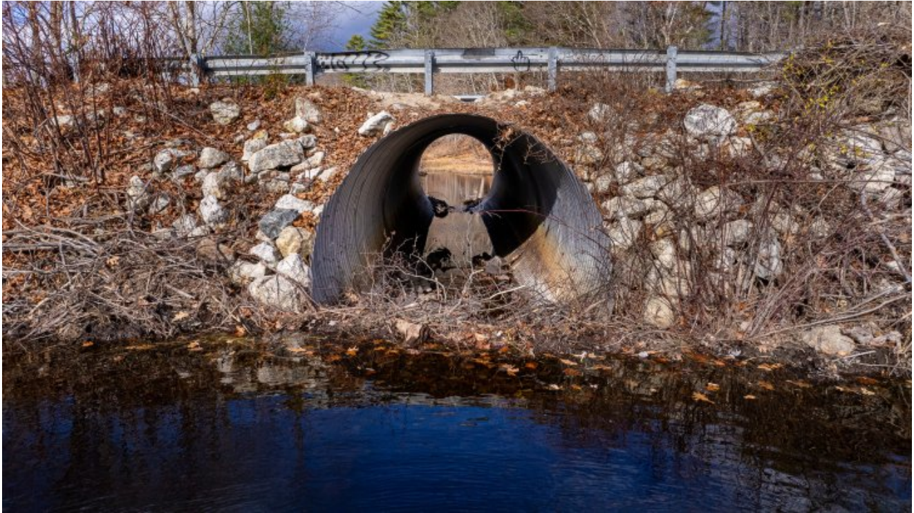
A rebuilt beaver dam is seen Nov. 7 at a culvert under Rabbit Valley Road in Oxford. The culvert connects a stream from Tripp Pond in Poland to Hogan Pond in Oxford. Russ Dillingham/Sun Journal Buy Image
