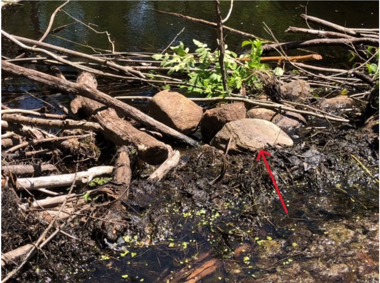
Rocks, some of them large and weighing an estimated 30-35 pounds, line the top of debris July 3, blocking the outlet at Tripp Pond and reducing water flow. Submitted photo
