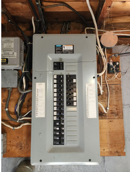
Main electrical disconnect
