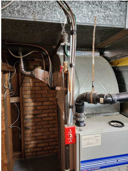
Main fuel shut off &amp; electrical disconnect
