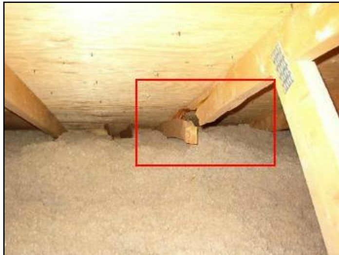
6. Top chord of truss is broken
