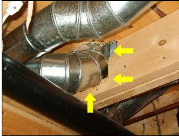
5. Joists are notched and weakened
