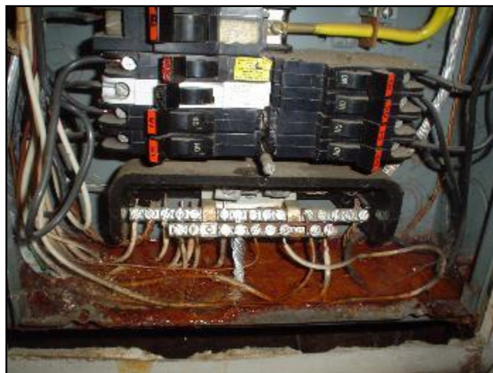
7. Water and rust in bottom of panel
