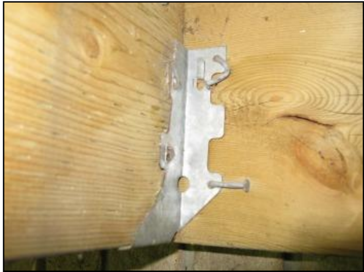
4. Poor end bearing, joist hanger connections
