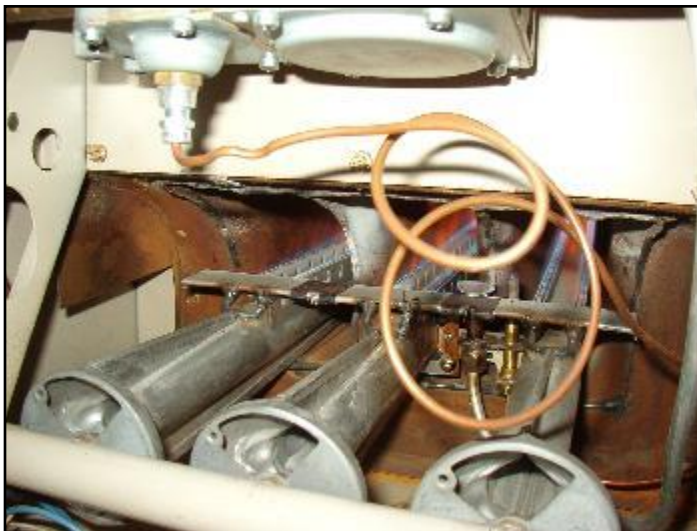
9. Rust at bottom of heat exchanger
