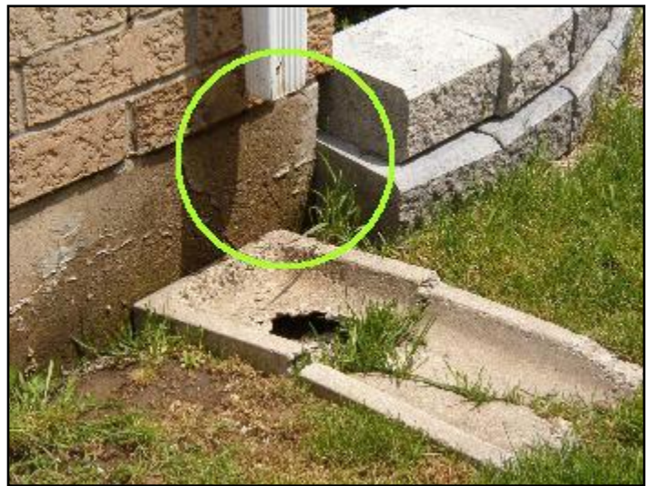
3. Downspout ends too close to building
