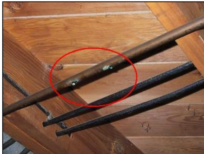
13. Leaking copper supply pipe
