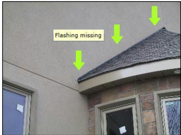
1. No kickout flashing at roof/sidewall junction
