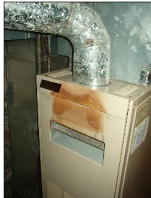
10. Evidence of furnace backdrafting
