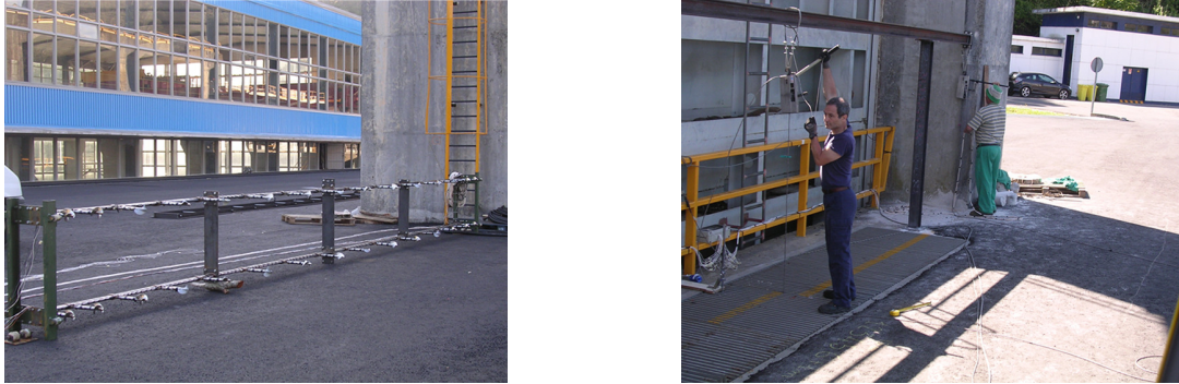
Fig. 6 – CM frame (left) and lifting winches (right)
