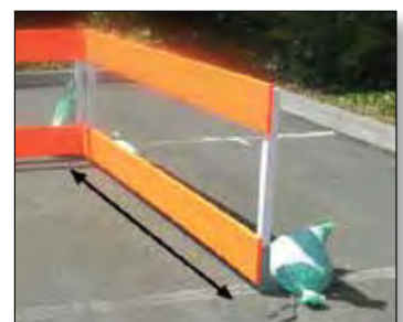
No part of the barricade protrudes into the walkway
