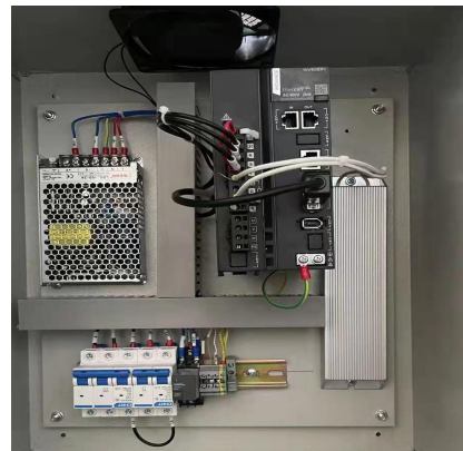
The internal arrangement of the electronic control cabinet is determined by the on-site project
