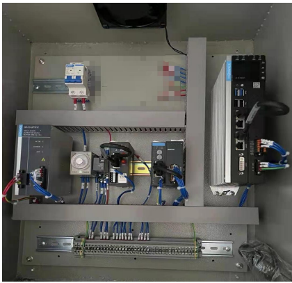
Fig. 4 Arrangement of electronic control cabinet
