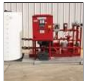
Diesel Pump Skids
