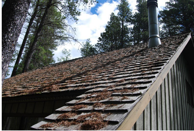
Figure 4: Example of a roof that has not been maintained well.
