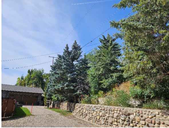
Figure 7: Trees growing in and around powerlines can be a fire hazard.
