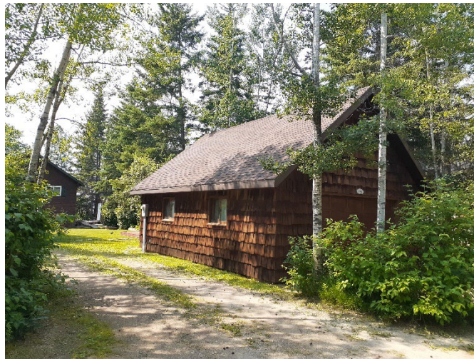
Figure 3: Homes with cedar shake siding provide little to no protection from wildfire.
