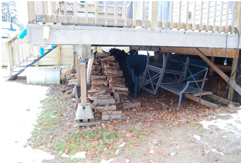
Figure 5: Accumulated materials underneath decks can act as an ignition source during a wildfire.
