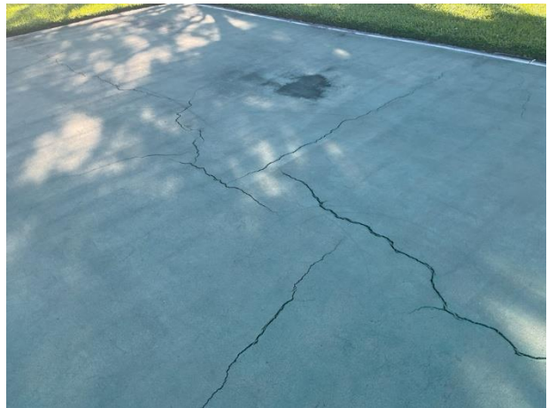
Surface cracks at basketball court
