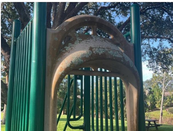
Playground equipment with biological growth
