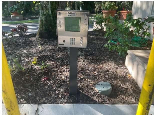
Gate entry keypad
