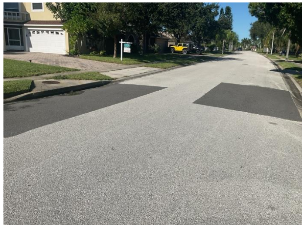
Pavement overview with previous repairs
