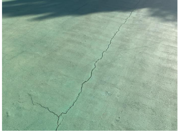
Surface cracks at basketball court
