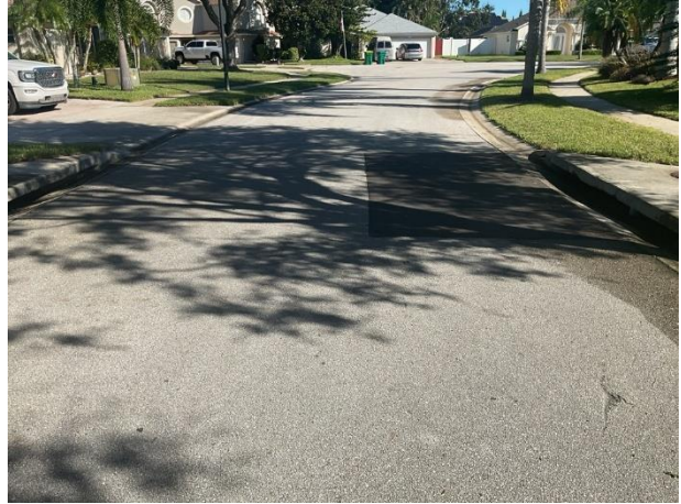
Pavement overview with previous repairs
