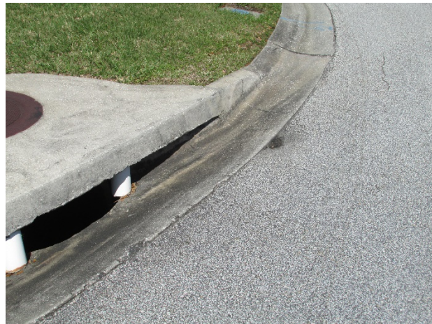
Catch basin with settlement evident on Sierra Drive
