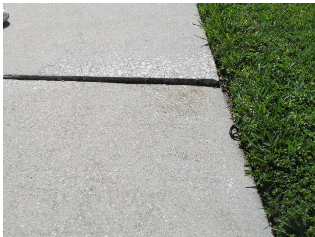
Concrete sidewalk with trip hazard evident
