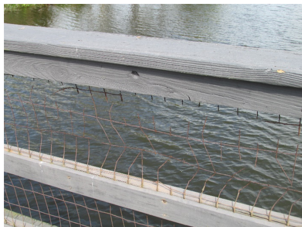
Bridge with rust and deterioration evident at railing wire mesh
