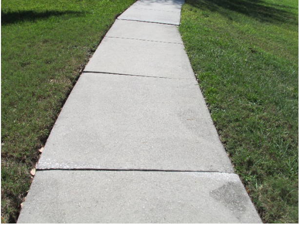
Concrete sidewalks with settlement evident
