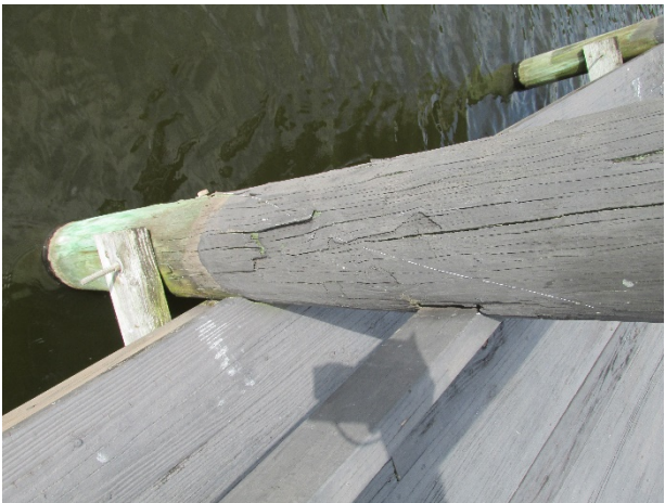
Wood piling deterioration evident
