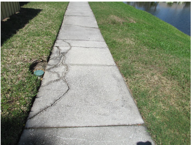
Concrete sidewalks with cracks and settlement evident
