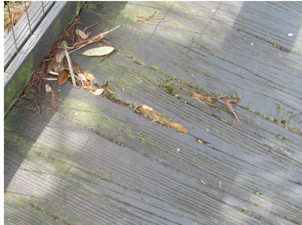
Bridge with wood deterioration evident
