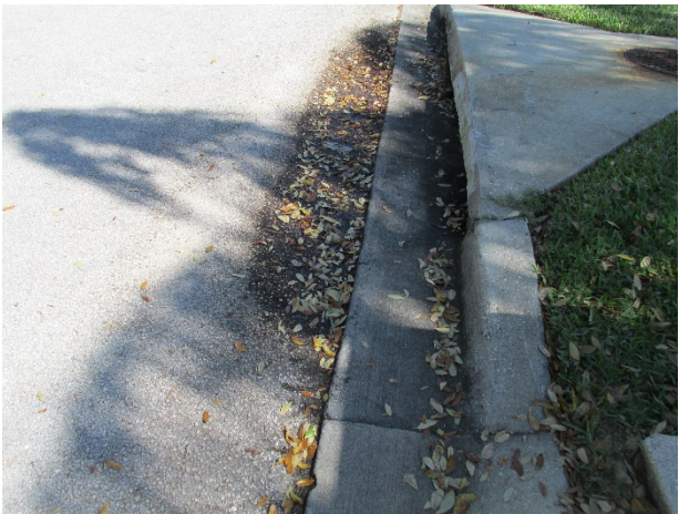
Catch basin with settlement evident on Sunward Drive
