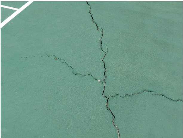
Tennis court cracks evident
