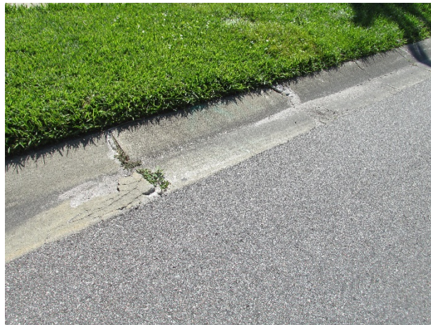
Concrete gutters with cracks evident
