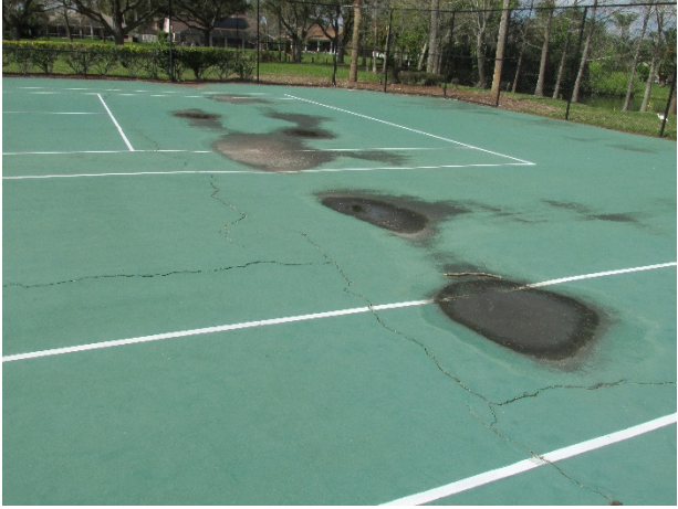
Tennis court surface settlement evident
