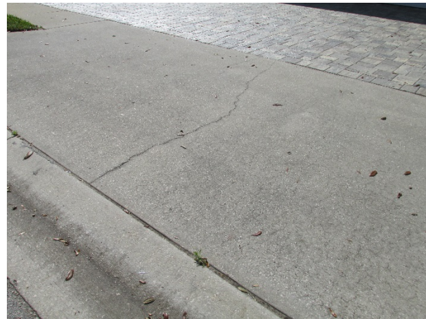
Concrete apron with minor cracks
