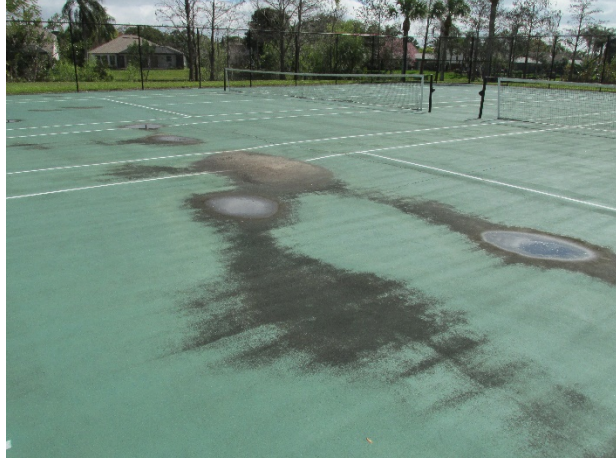
Tennis court surface settlement evident
