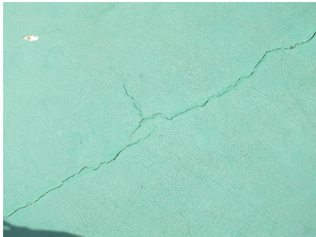
Basketball court cracks evident
