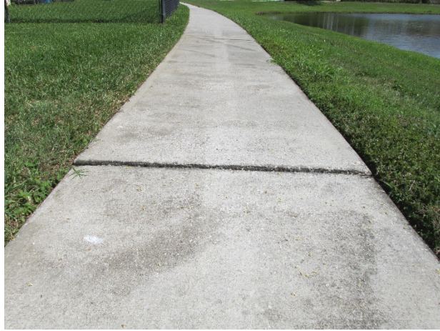
Concrete sidewalk with trip hazard evident
