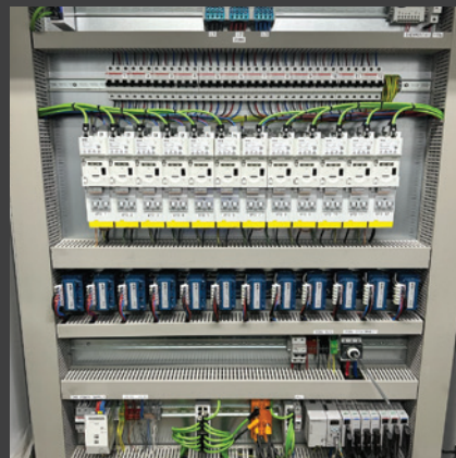
Custom Wiring & Controls
