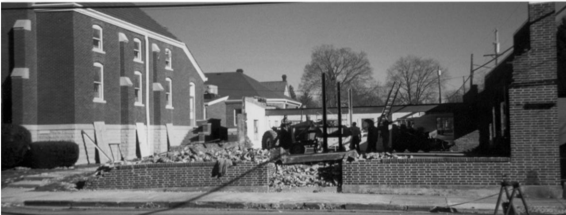
Photo above: “And the Walls Came a Tumblin’ Down!!!” Ed Keiter, John Dailey, Sam Murphy, Charlie Lakatos and Mike Keiter work to remove the old Kirk Music building to open up the view of the south side of the church building and to create more parking.
