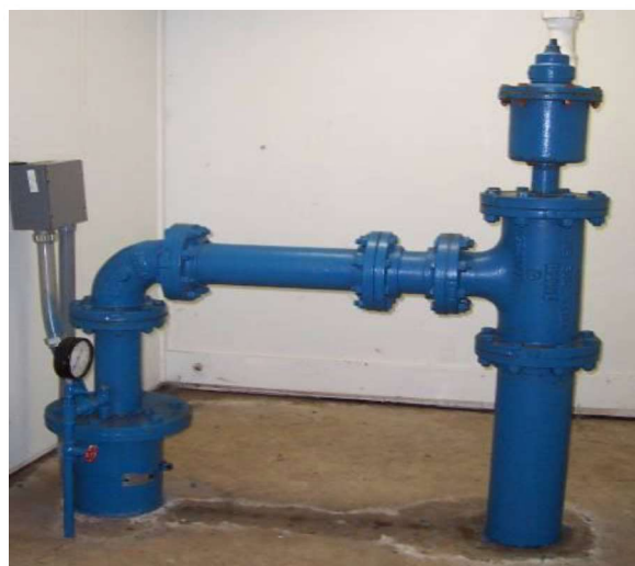
Mechanical Equipment for Well 7
