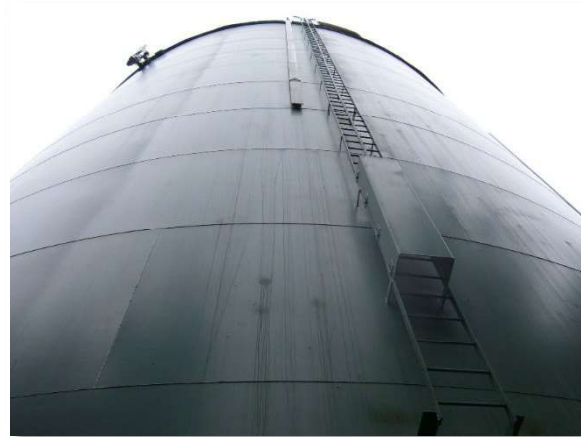
California Avenue Tank No. 2
