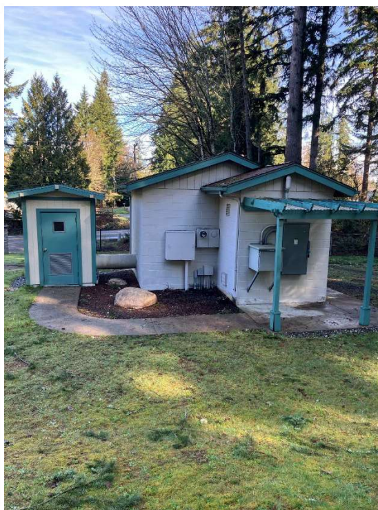
Well 9 Building and Treatment Building
