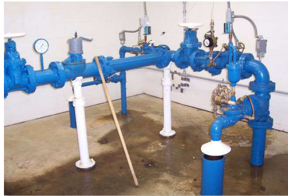
Well 10 and 11 Interior Piping
