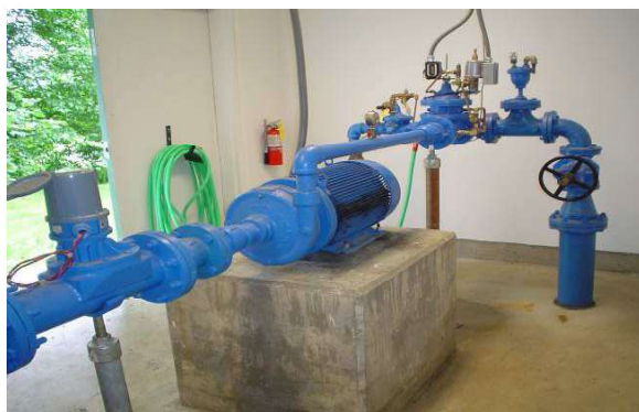
Banner Road Booster Pump Station
