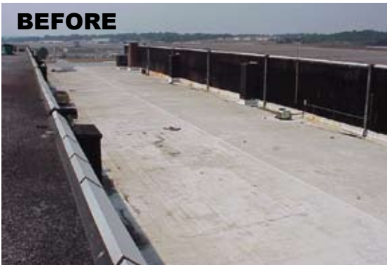
These three photos (above and below) show stages in the re-roofing of one of the facility's three service bays. Above, the roof area is shown before a slope build-up structure is added for better drainage.
