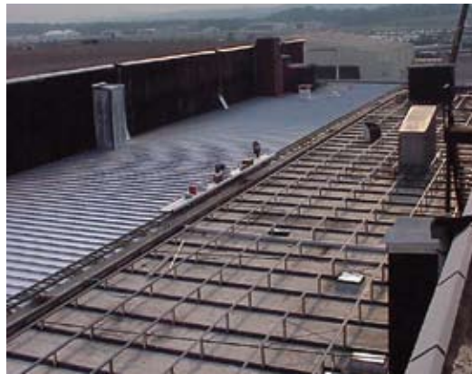
To cut labor costs, the erector created a roller system that allowed workers to move materials across the roof quickly and efficiently. The platform shown below carried bundles of panels to the roofers in minutes.
