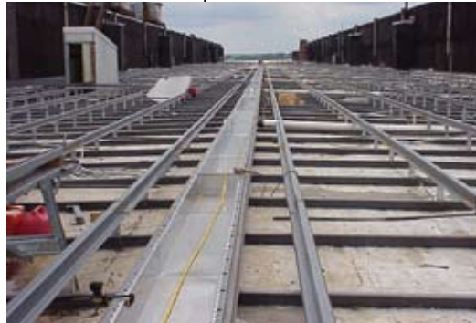
The detail photo left shows a close-up of the new gutter running through the center of one of the service bay areas. No welding was allowed on the roof during the retrofit. Welds were factory made.
