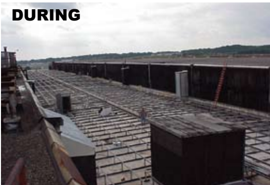
In the photo to the left, the slope-build-up structure has been added, ready for the new roof panels. In the photo below, the new panels are in place. The groove running through the center of the recessed area is a new gutter to drain the area.
