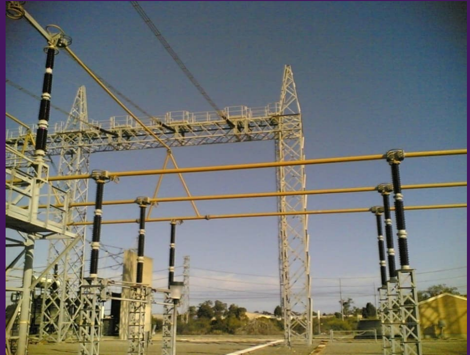
Ref [1] Western Power Northern Terminal 330kV Gantry
