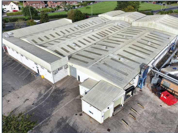
Figure 2. Low oblique image of a factory industrial unit from a drone roof survey and roof inspection in Yorkshire, UK.
