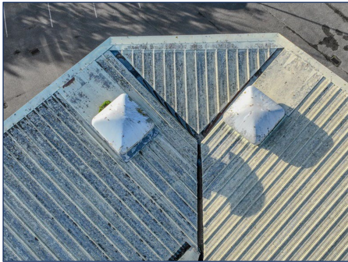
Figure 5. Corner detail of industrial roof with valley gutters showing slight sign of corrosion from a roof survey and inspection, in Yorkshire, UK.
