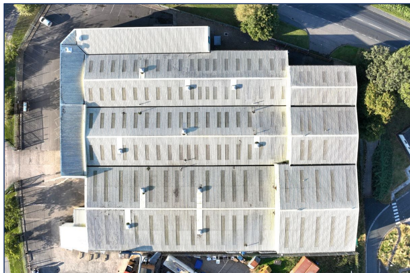
Figure 1. Nadir image of industrial unit with trapezoidal roof on portal framed building with 6 valley gutters. Yorkshire, UK.
