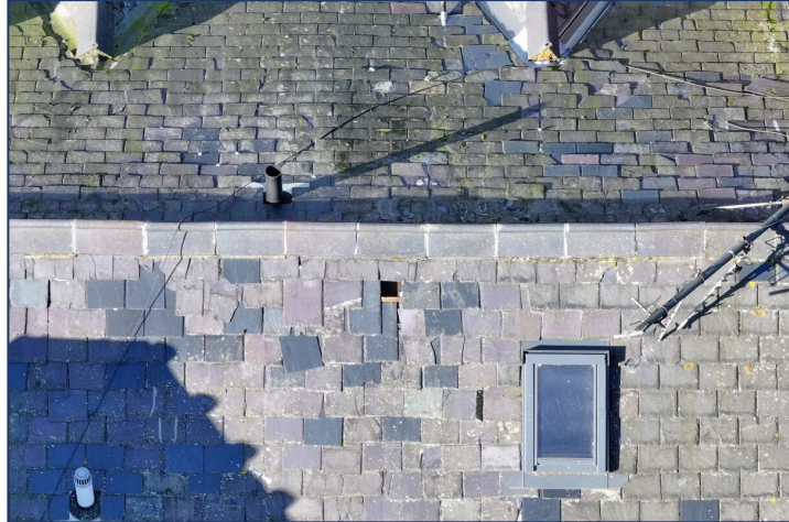
Figure 4. This image was taken 35 metres above the property, showing a hole in the roof caused by a missing slate.
