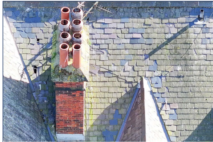
Figure 3. Holes in the slate roof and many slates that were broken or displaced.
