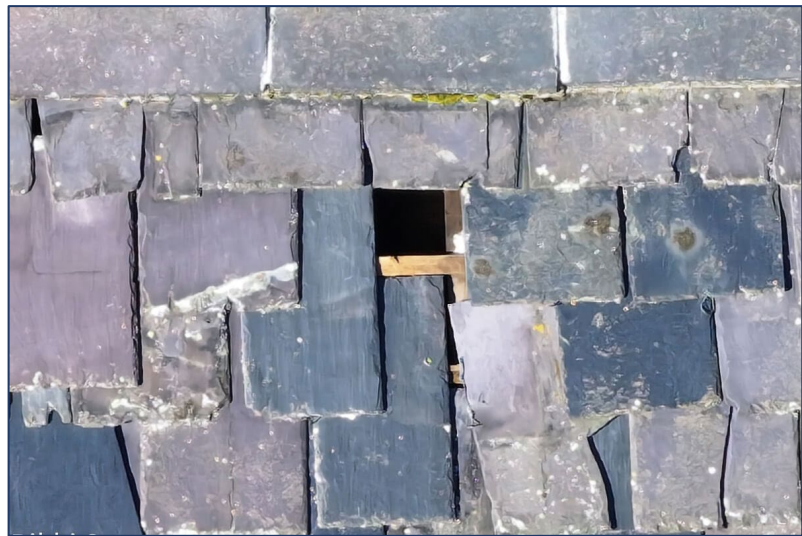
Figure 5. Zoom x 10 image of hole in roof, showing roofing lath underneath and part of a roofing truss.
