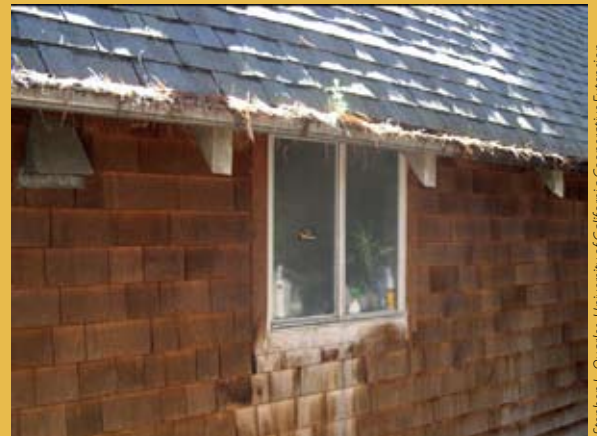
Accumulated fuel in rain gutter.
