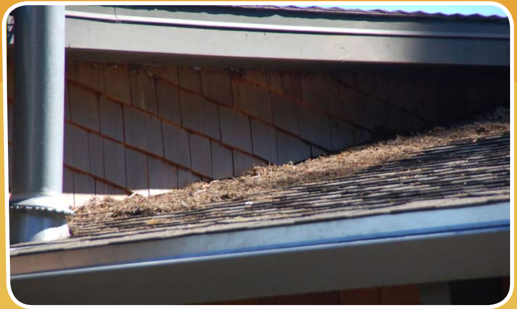
Accumulated pine needles on this complex roof could allow embers to ignite roofing materials.
