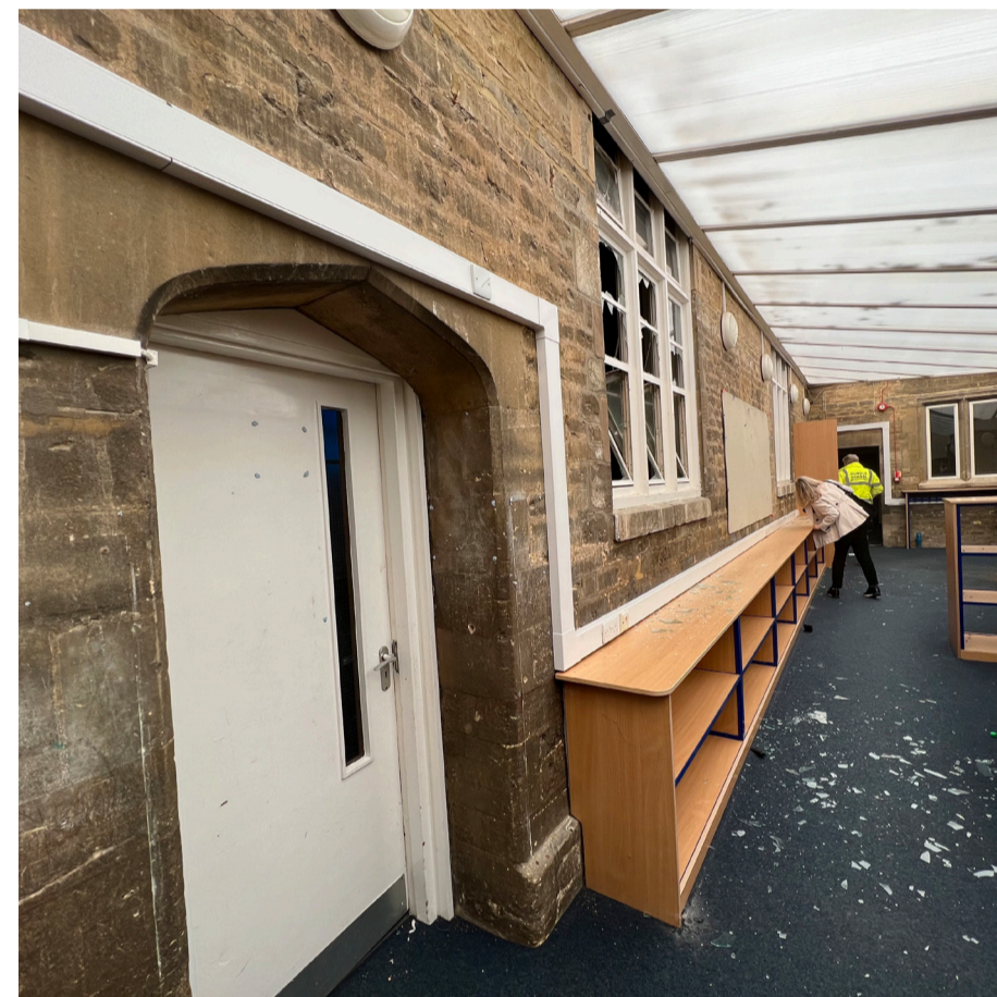
View 3 - interior view showing the typical damage to the original stone features of the building
