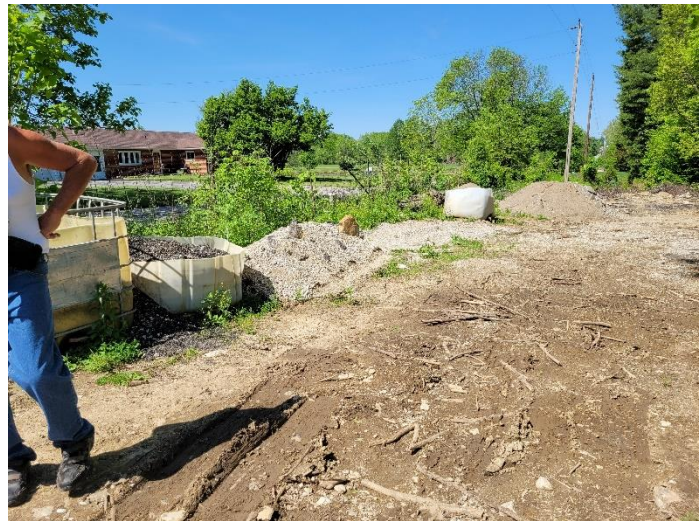
Picture 90 – Containers of crushed asphalt/rock and sand stockpiles For drive maintenance and filling in wet areas
