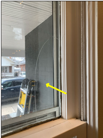
North dining area window cracked but operational.
