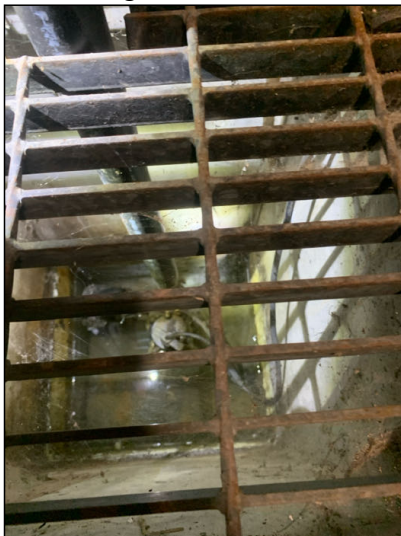
Foundation Sump Pump
