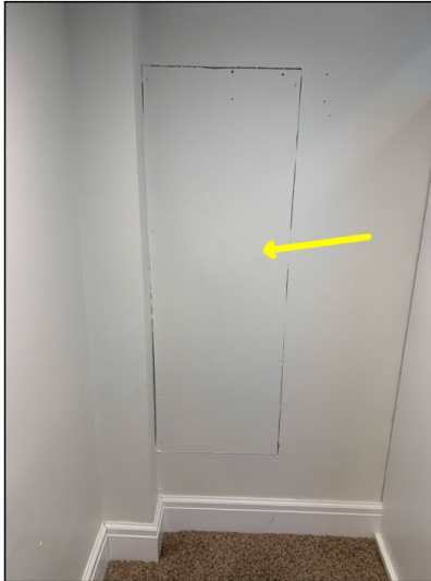
Plumbing access for bathroom shower.
