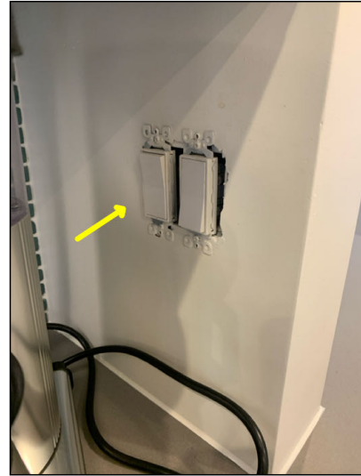
Switch on the left is for the Sink Disposal
