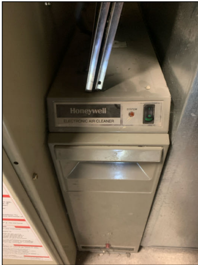
System does not appear to be functional at time of inspection.
