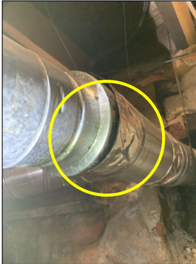
Needs to be re taped and sealed. Safety issue with exhaust fumes in home
