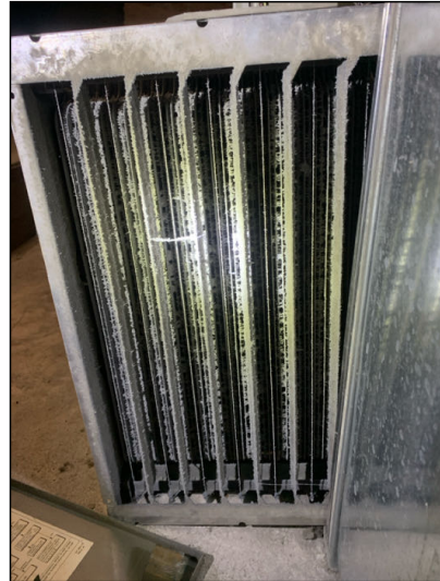
This system has a Electronic filtration system. This is the filter and needs serviced. Contact a certified HVAC professional for examination.
