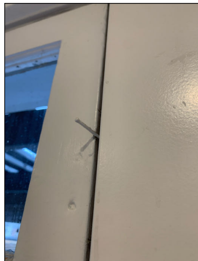
Nail is holding window above Patio door closed. Window is missing latch. Recommend add latch.
