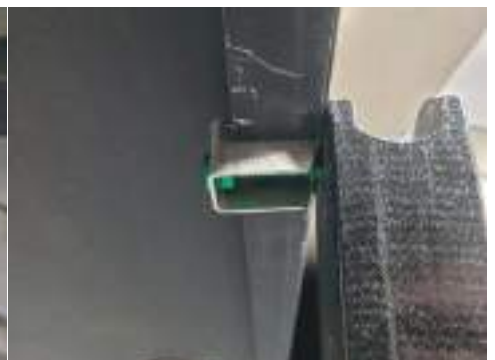
Figure 18: IR Ballast frame connection to solar panel
