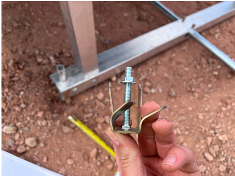
PHOTO 13: Bracket deformation after testing
