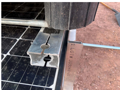
PHOTO 7: Slight deflections noted under load
