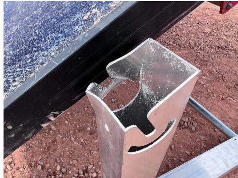
PHOTO 14: Upright mount deformation after testing
