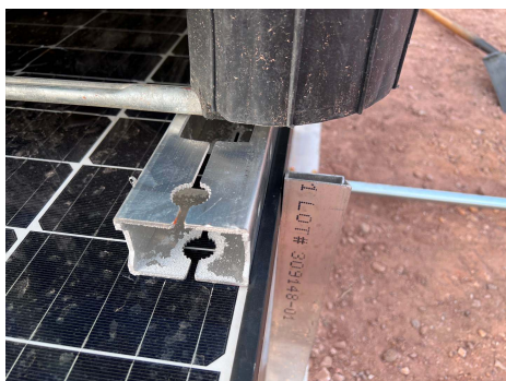
PHOTO 7: Slight deflections noted under load
