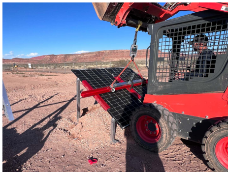
PHOTO 4: Test setup with dynamometer and chains connected
