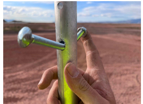
PHOTO 6: First anchor pullout with drilled thru hole deformed
