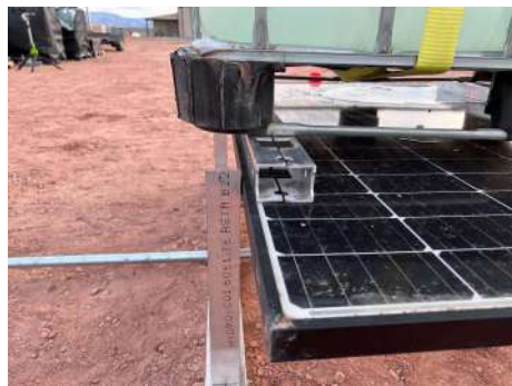
PHOTO 8: Slight deflection noted under load
