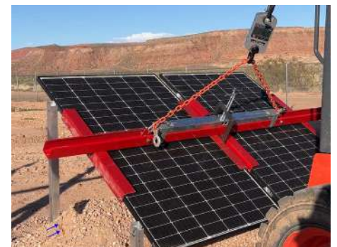
PHOTO 9: Test 2 - Evidence of ballast shift
