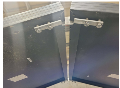
Photo 6: Brackets below solar panel at top point of the IR-EW15 frame
