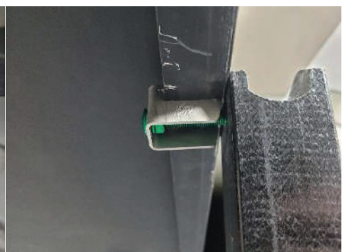
Figure 18: IR Ballast frame connection to solar panel
