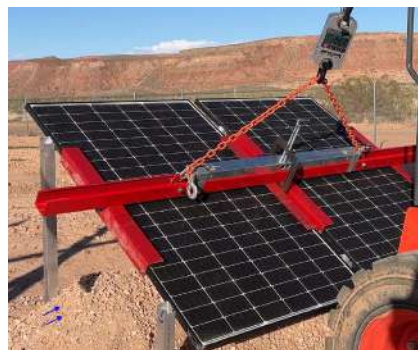
PHOTO 8: Test 2 - Evidence of ballast shift
