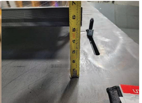
Figure 6: Height from roof to panel, Runs 2 & 3
