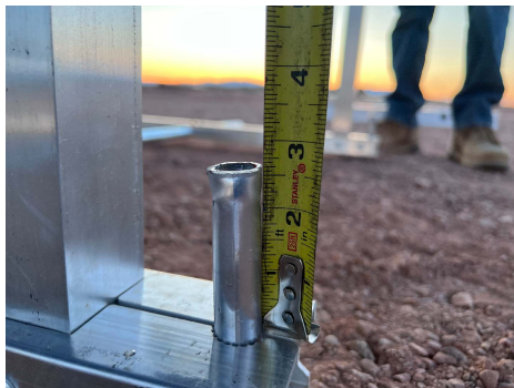
PHOTO 4: 'Stickout' measurement example at Spike #3
