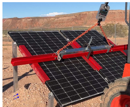
PHOTO 8: Test 2 - Evidence of ballast shift
