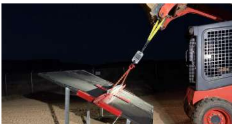
PHOTO 7: IR-30 Solar Racking System at max load
