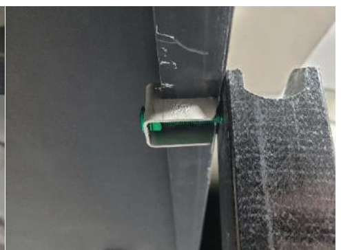
Figure 18: IR Ballast frame connection to solar panel
