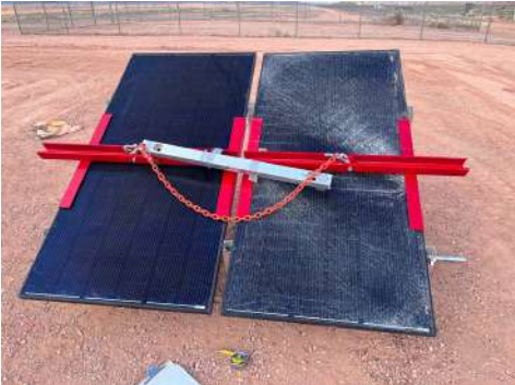
PHOTO 10: Solar panels after testing
