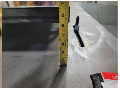
Figure 6: Height from roof to panel, Runs 2 & 3
