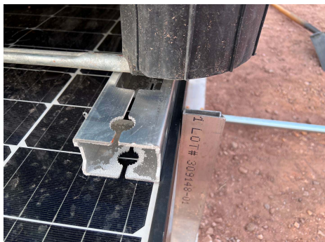
PHOTO 7: Slight deflections noted under load
