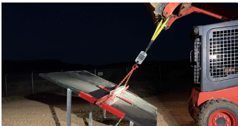
PHOTO 7: IR-30 Solar Racking System at max load
