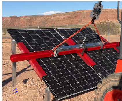
PHOTO 8: Test 2 - Evidence of ballast shift
